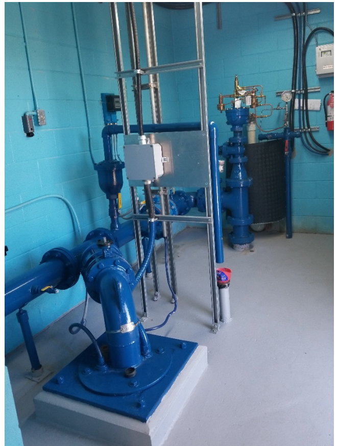
Inside the Lodge Road Pump House
